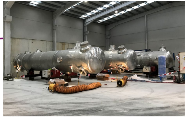
Primary Circuit Heat Exchangers
